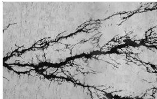
Figure 2: Shape of CSCC Crack
